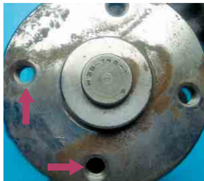
Damage at the stud bolt ends
